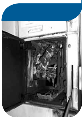
Chinatown exchange fire damage
